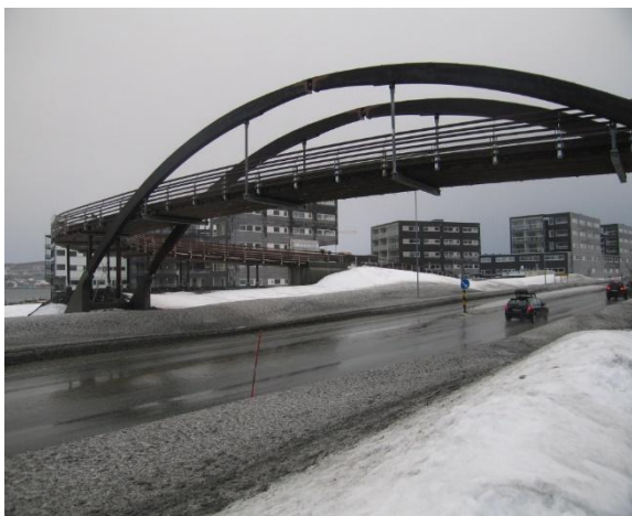
Figure 8: Arch Bridge with deck type "SLTD" at Tomasjord, near Tromsø, Norway. Note the horizontal curvature of the deck.
